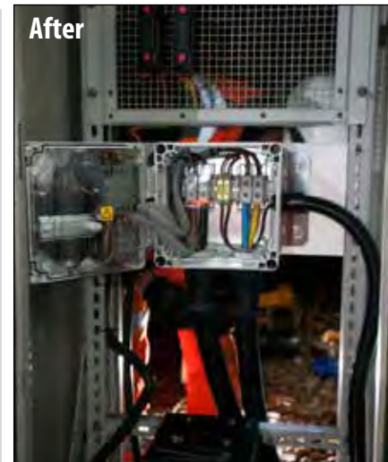
New and old cable. Legacy Al cable on the right interfacing with new Cu unarmoured cable on the left
